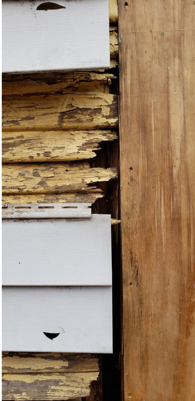
Request #2 – Photo of existing vinyl siding and wood siding beneath. Photo submitted by applicant.
