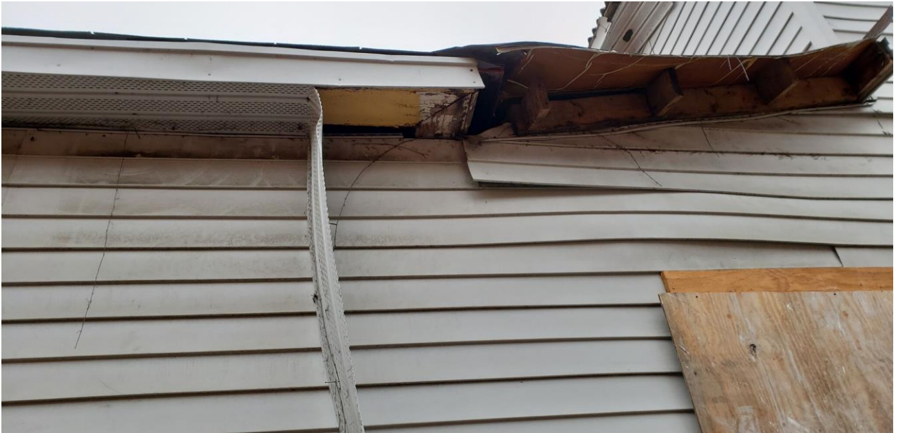
Request #s 2 and 3 – Photo submitted by applicant showing current vinyl siding and cornice.
