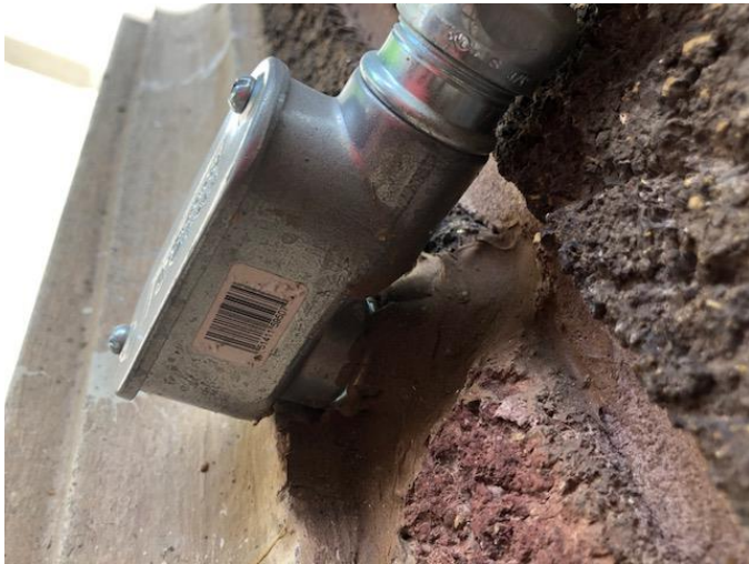
Close up views of security camera and car charger hardware installed
