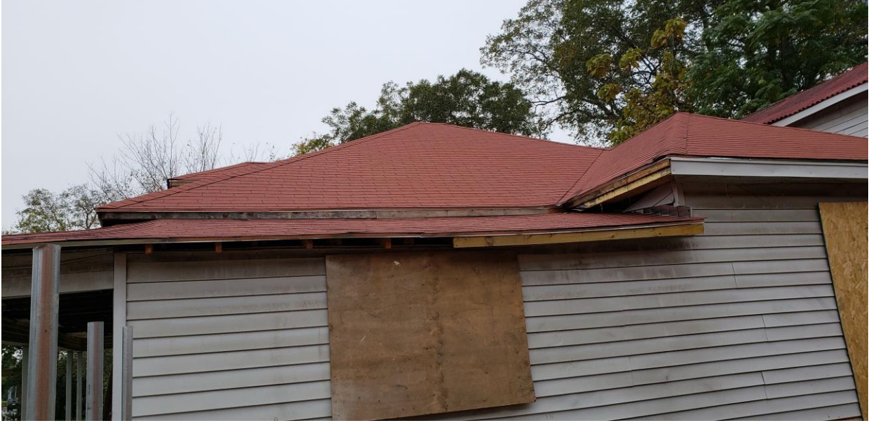
Request #s 2 and 3 – Photo submitted by applicant showing current vinyl siding and cornice.
