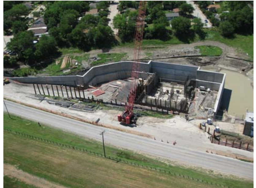
Pavaho Pump Station - 2006 Bond Program
