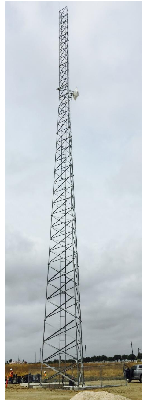
180-foot Communications Tower at Joint Booster Pump Station 3
