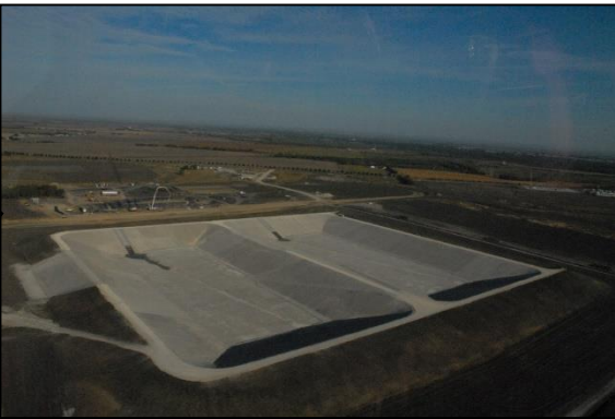
JB3 Pump Station Suction Reservoir
