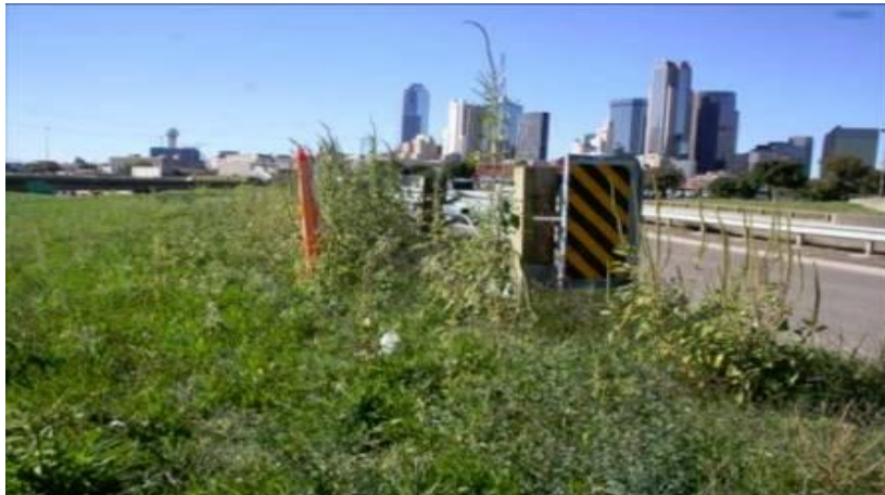
Overgrowth around guardrails
