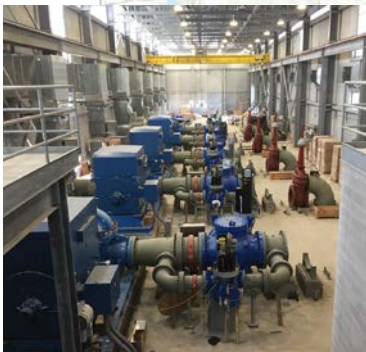
Joint Booster Pump Station 3 (JB3)
