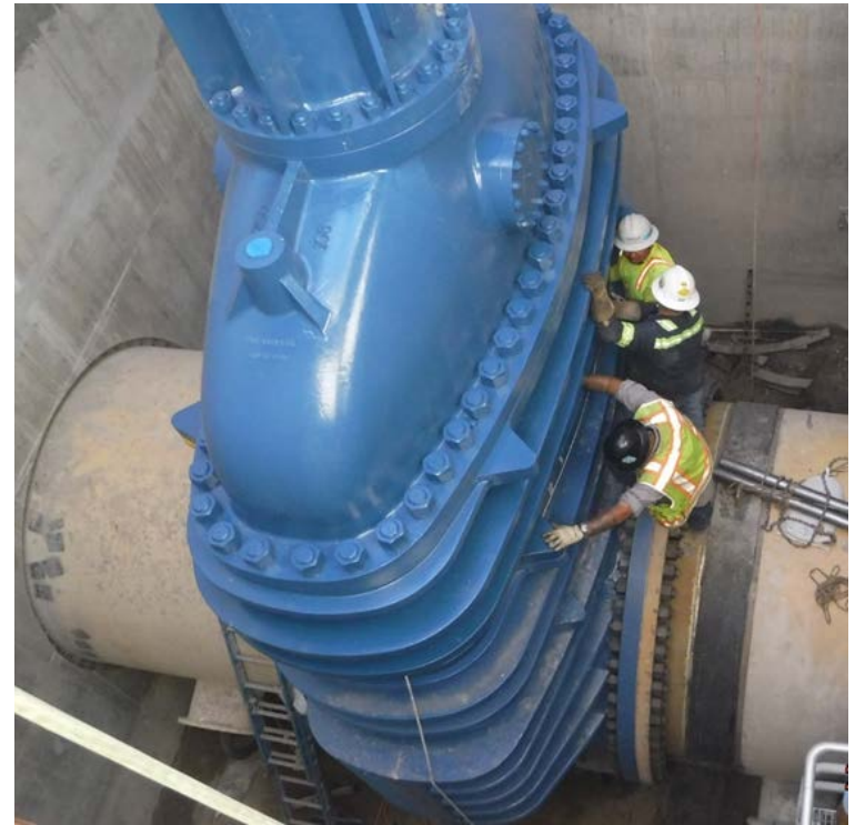
108" Gate Valve at Midlothian Balancing Reservoir
