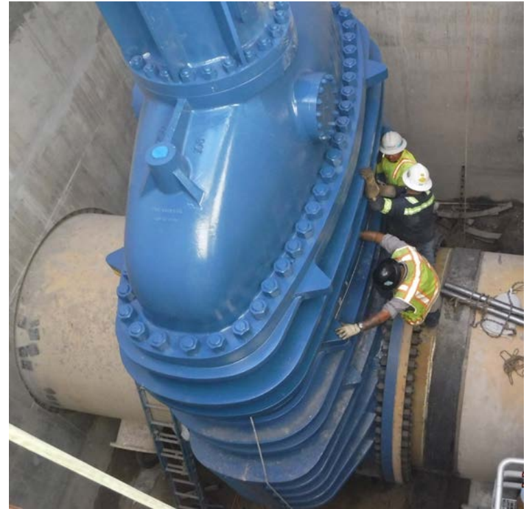
108" Gate Valve at Midlothian Balancing Reservoir
