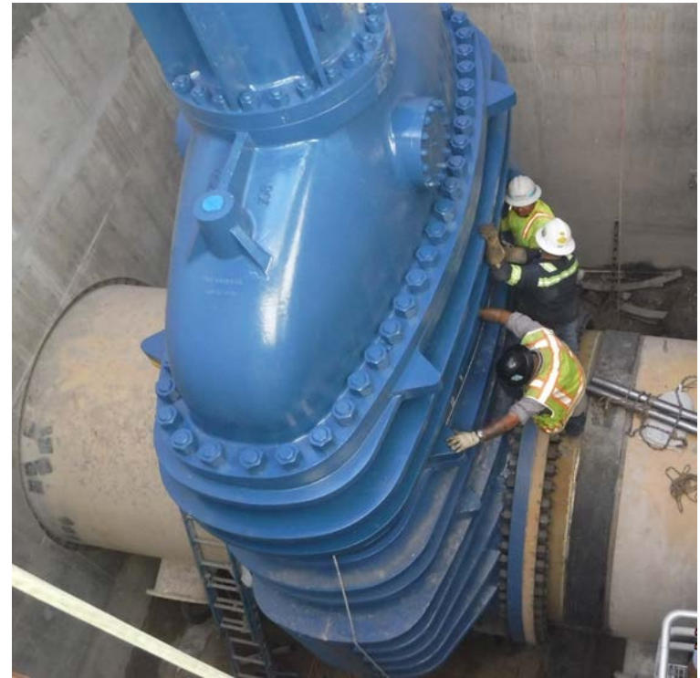
108" Gate Valve at Midlothian Balancing Reservoir
