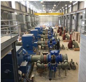
Joint Booster Pump Station 3 (JB3)
