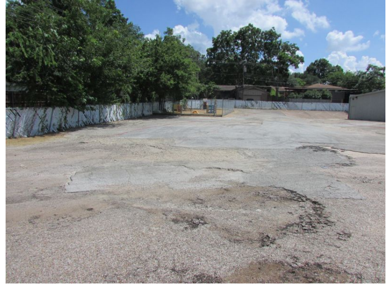
Deteriorated site conditions
