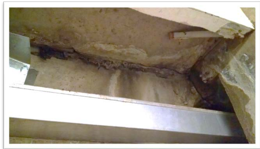
City Hall water infiltration
