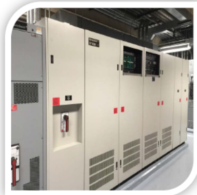
City Hall's Critical Power System was at "end of life" in 2012 - parts are increasingly difficult to find
