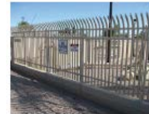
Impasse II Security Fencing
