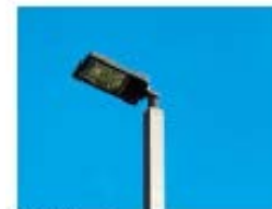
LED Light pole
