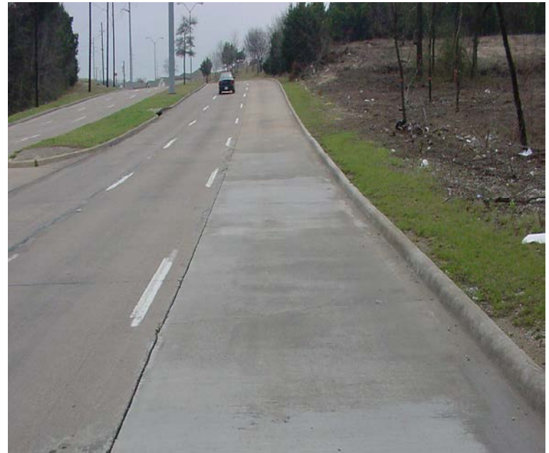
Full lane replacement required by ordinance
