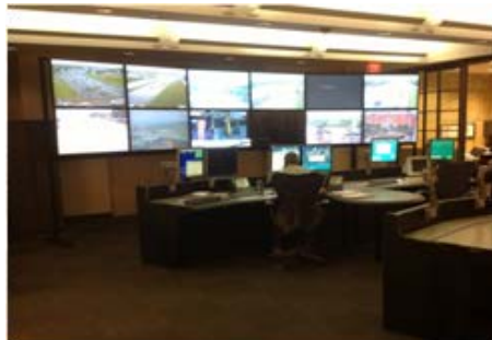
Central Computer System
