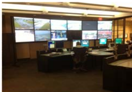
Central Computer System
