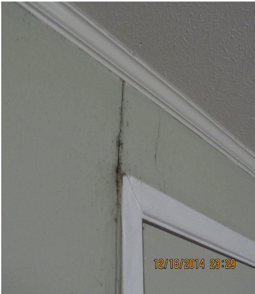
Evidence of Bed Bug Infestation on Walls
