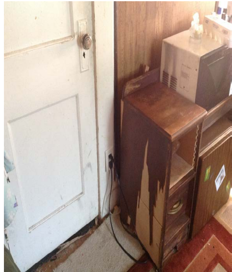
Electrical Violation Abated
