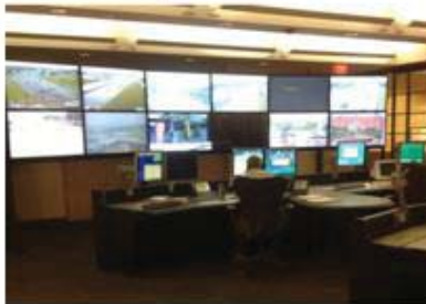
Central Computer System
