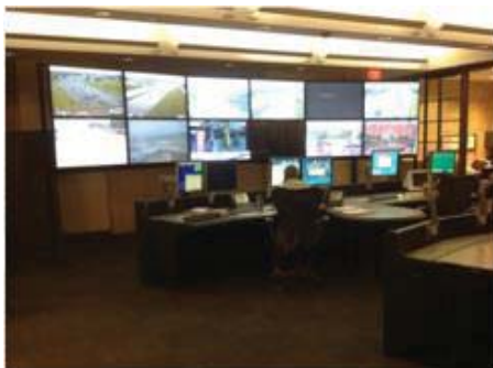
Central Computer System
