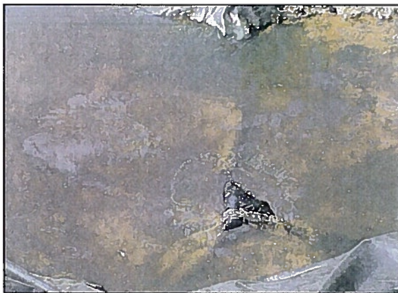
Figure 3: Petroleum LNAPL observed on top of water present inside an excavation.
