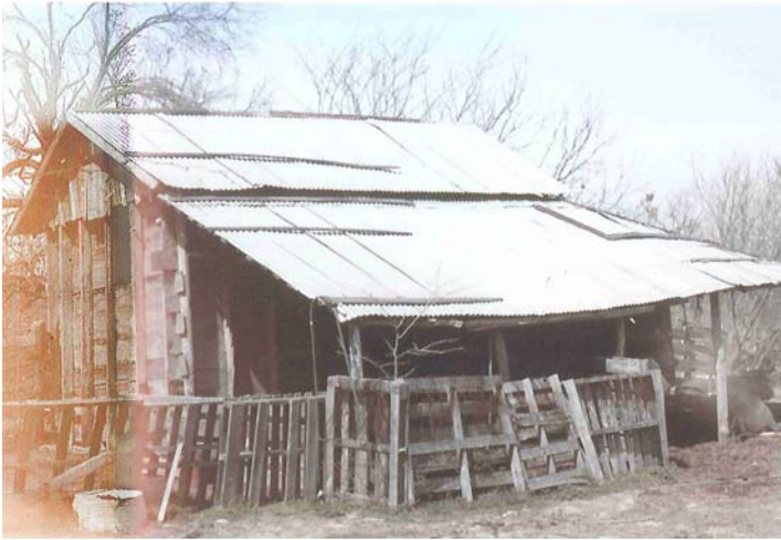
Figure 12 - Plank barn, March 1973, shows barn's appearance prior to collapse. Photo by Architect William Thomas Odum
