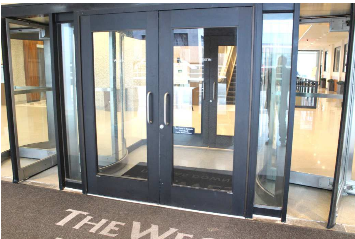
Typical existing building entry (unmodified during rehabilitation) (top), January 2017 Ground level hotel entry at northwest showing added interior doors to create vestibule (bottom), January 2017
