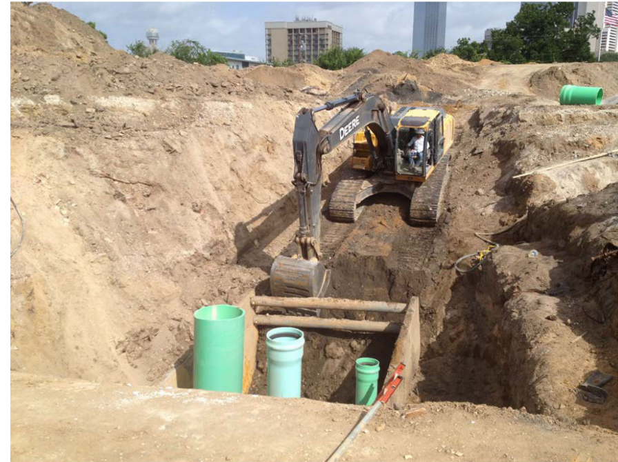
MULTIPLE SIPHON LINES
