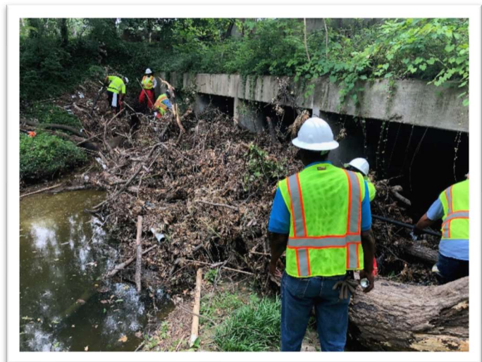
Credit: Dallas Water Utilities
